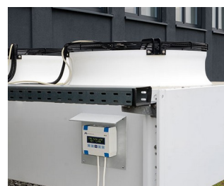
Heating/air conditioning/ventilation control
