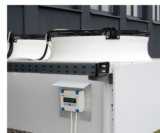
Heating/air conditioning/ventilation control
